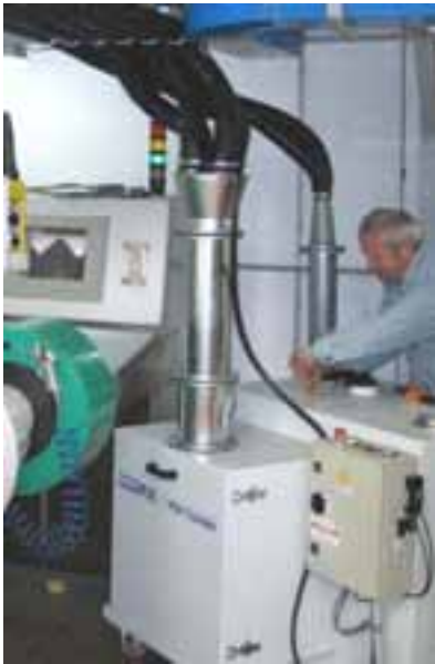
Web Cleaner installation
