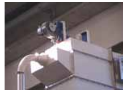
DA 600 on static separators
