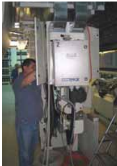
ESA ACE Rotostatic installation
