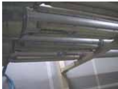
Clear Tube instalados
